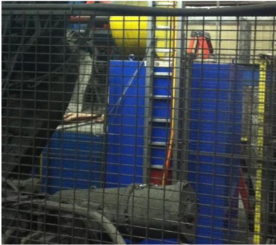
Interpower Induction 10 kHz heater installed at Walker Forge
